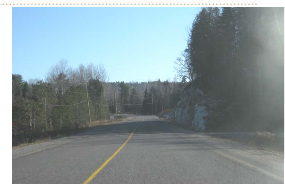
Newly constructed section (2007) - Wider platform (lane and shoulders) - Good visibility (no hazards)
